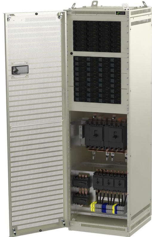
Rectifier 54 kVA + 48 kW B-input (without front covers)
